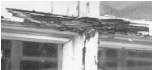
A typical example of a lack of planned maintenance now requiring replacement on a school
